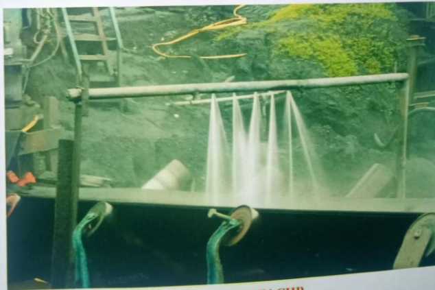
MIST SPRAY IN CHP
